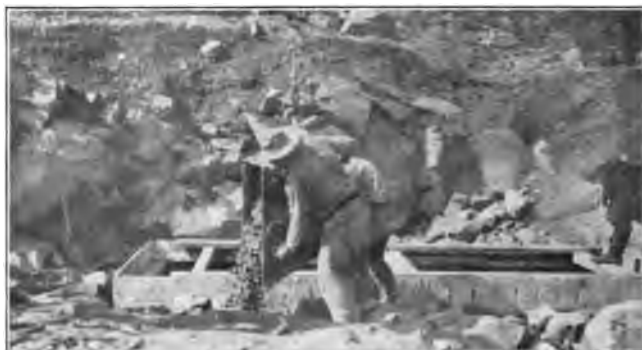
A. MAKING CONCRETE COLLAR, NEW SHAFT AT NORTH LAKE MINE, 1912, ONTONAGON COUNTY.
